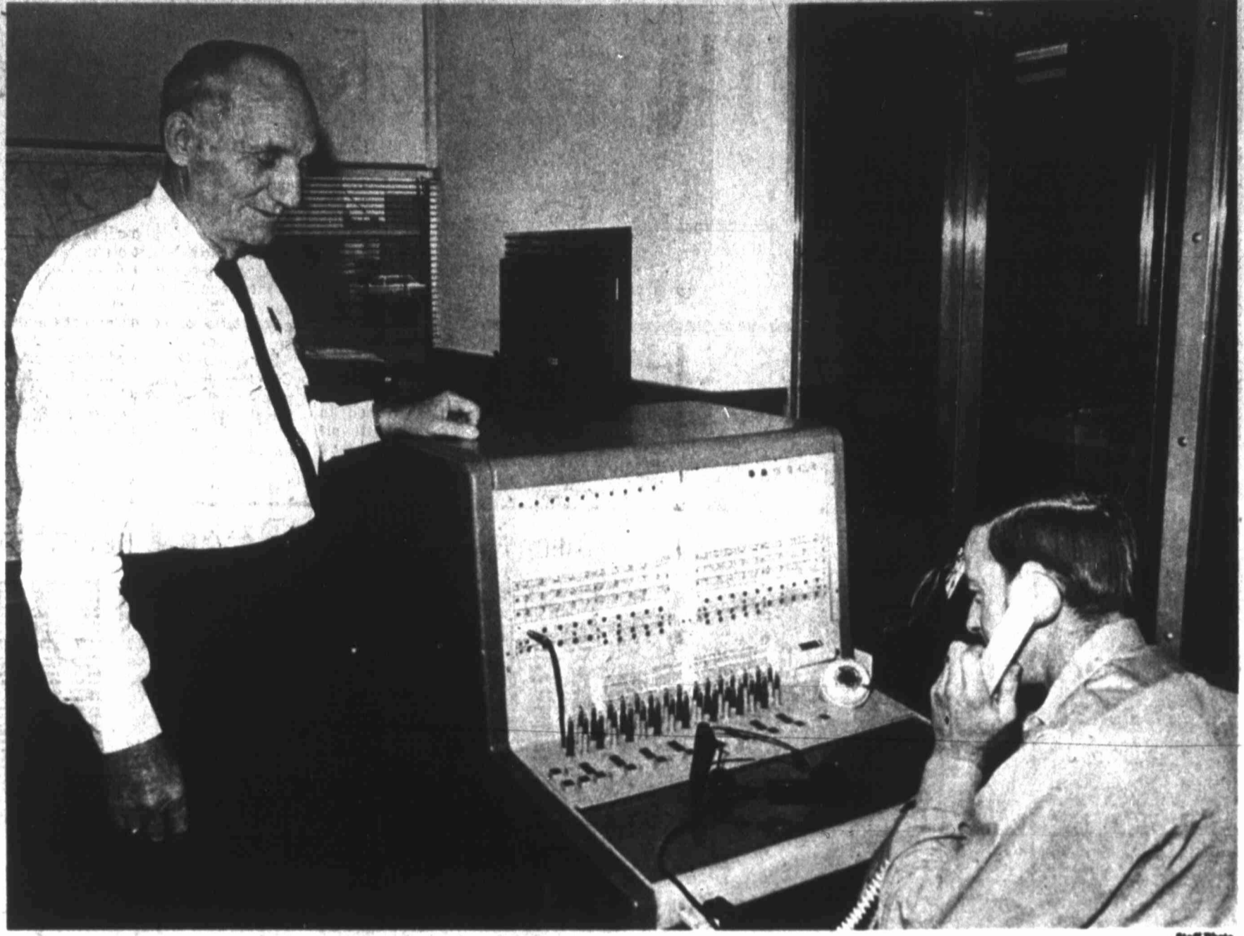
Midland Fire Chief Melvin Little, left, and fire dispatcher John Shumake run the new emergency services master switchboard through a practice session. It becomes operational in three days.
