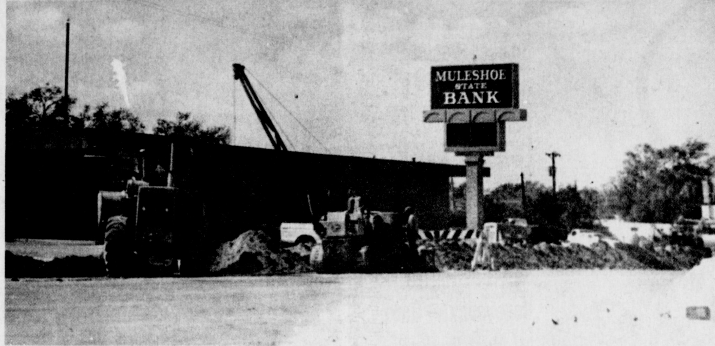
MOVING UTILITIES FOR CONSTRUCTION . . . The city began this week moving water lines along Highway 84 in preparation for the widening of U.S. Highway 84 in Muleshoe. Water lines were dug up and relocated this week providing for some aggravation to motorists on the highway. This phase of construction and relocation should be completed soon.
