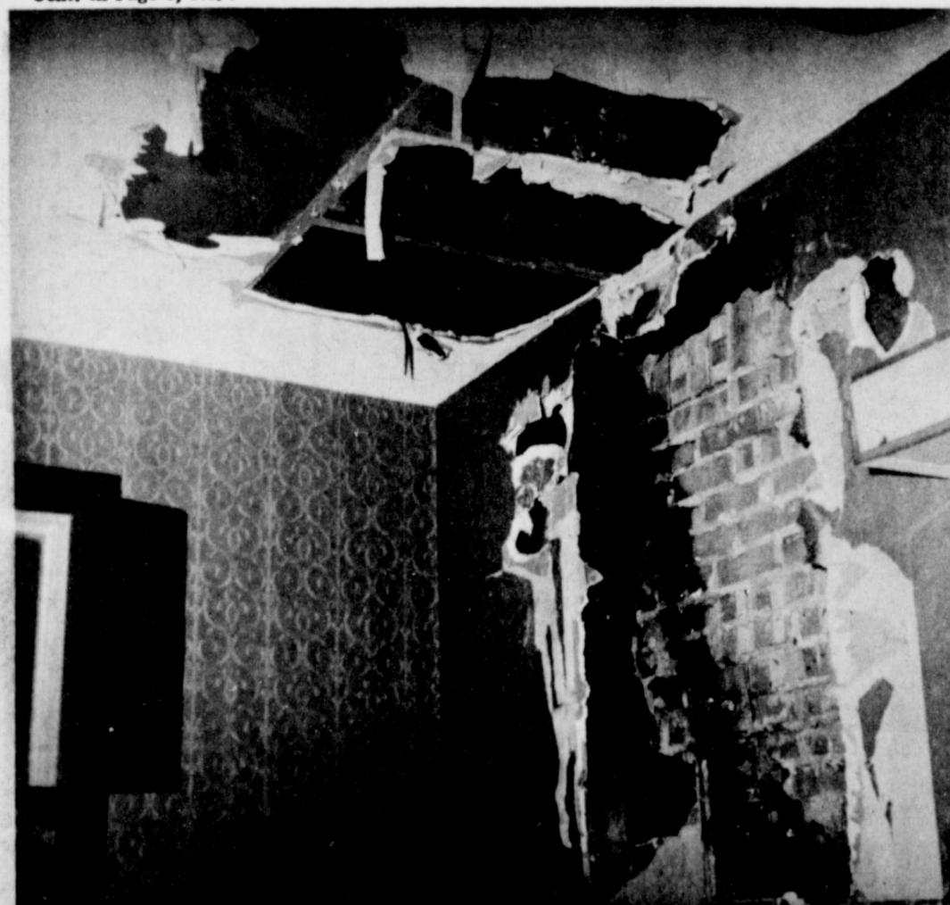
FIRE DAMAGES HOME . . . The home of Mr. and Mrs. Dick Johnson, 1810 West Avenue C, was damaged by fire Sunday night. This picture shows the master bathroom that was heavily damaged when a gas heater apparently overheated, causing the wall to go up in flames. Local units of the Bailey County Volunteer Fire Department were rushed to the scene about 9:30 p.m. and the blaze was quickly extinguished.
