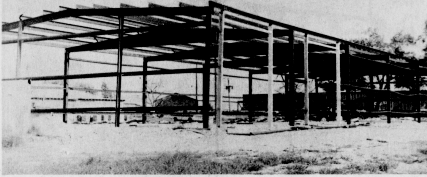
NEW CITY BARN . . . The new City Maintenance Barn and Shop is now under construction on Highway 84, near the east city limits. City Manger Albert Field reports that the new building should be completed in two to three weeks. Workers should be
