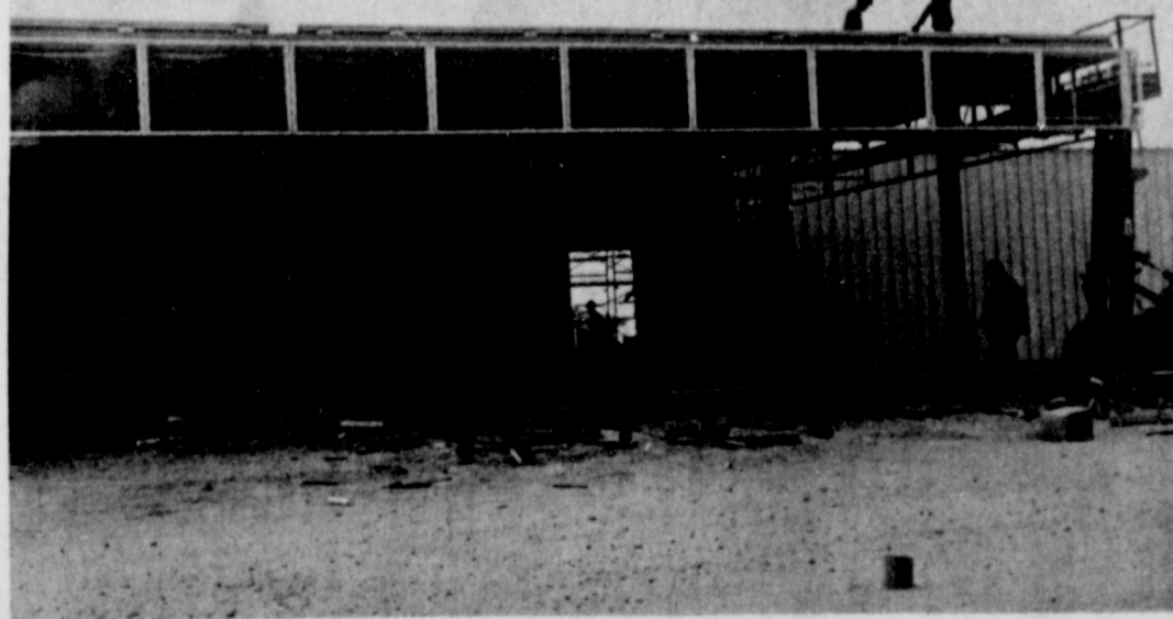
NEW FORD HOUSE GOING UP . . . Siding has been put on the sides of the metal frame building that will soon be the new home of Muleshoe Motor Company. Construction is progressing very rapidly on the new building and it shouldn't be too long before the building is completed and the Ford Company's place of business changed from the Crossroads to this new location on West American Blvd.
