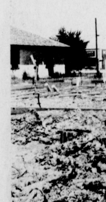
CONSTRUCTION UNDERWAY...Construction has begun on the new Dairy Queen which is being constructed in Muleshoe. The building is being built on the corner of Twelfth Street and American Blvd. Company executives report that the construction will be completed and the Dairy Queen open for business by the first of October. The family dining place will have both drive-up and walk-up windows, plus a dining room that will seat 60 people.
