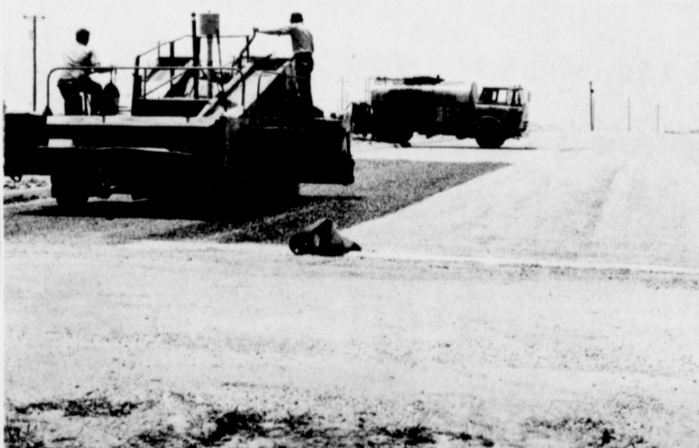
PAVING STARTS ON NEW STREET...The new residential section of Muleshoe under construction near Eighth Street and Avenue G is getting a new paved street. The street is being paved by the land developers with Jake Diel Dirt and Paving doing the construction work. Several new homes are presently under construction in this area.
