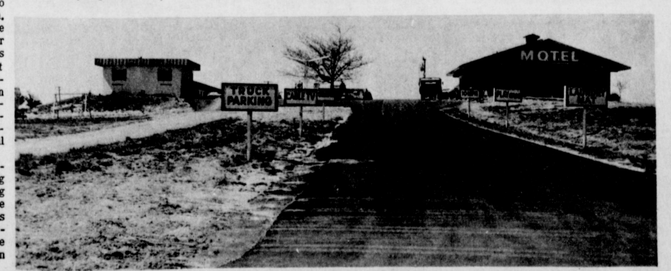
MOTEL UNDERGOES REMODELING...The Muleshoe Motel on the west end of American Blvd, has undergone several changes in the past months. The rooms have been completely redone and redecorated, the motel office has new siding on it plus a large new
