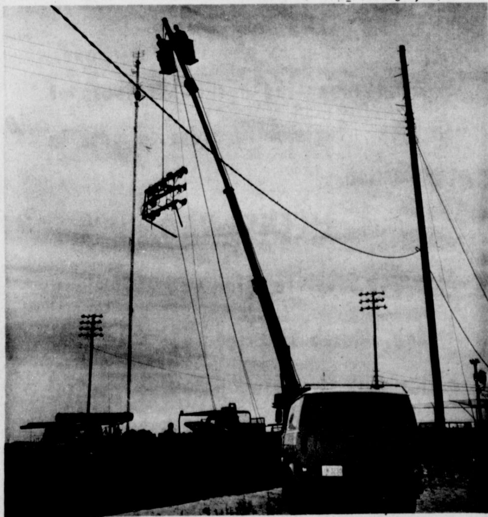
BABE RUTH PARK INSTALLS LIGHTS...New lights went up at the Babe Ruth Baseball Park this week after improvements were approved by the Muleshoe City Council recently. The Park Ruth Tournament which will be played in Muleshoe this year. The lights were installed by Southwestern Public Service employees.
