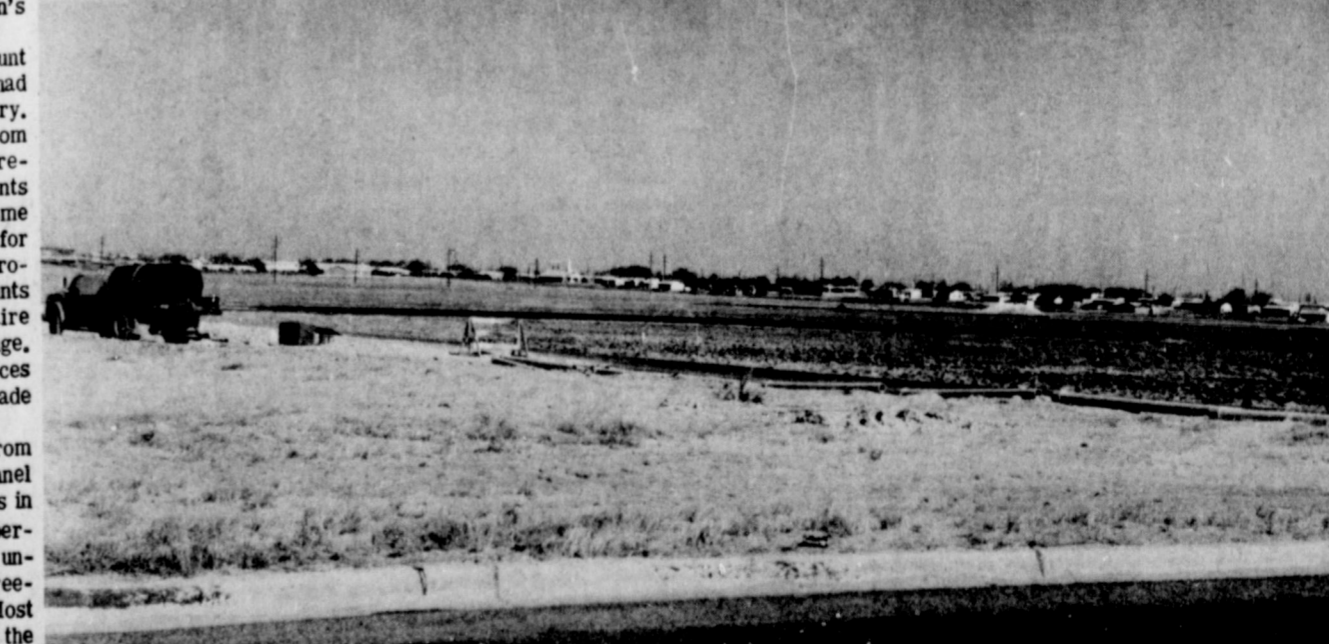
WORK CONTINUES ON PARK ... Construction on the new Muleshoe City Park on West Avenue D is coming right along. Grass park including a Youth Football field, softball field, restrooms and park equipment. The city has applied for matching funds of $25,000
