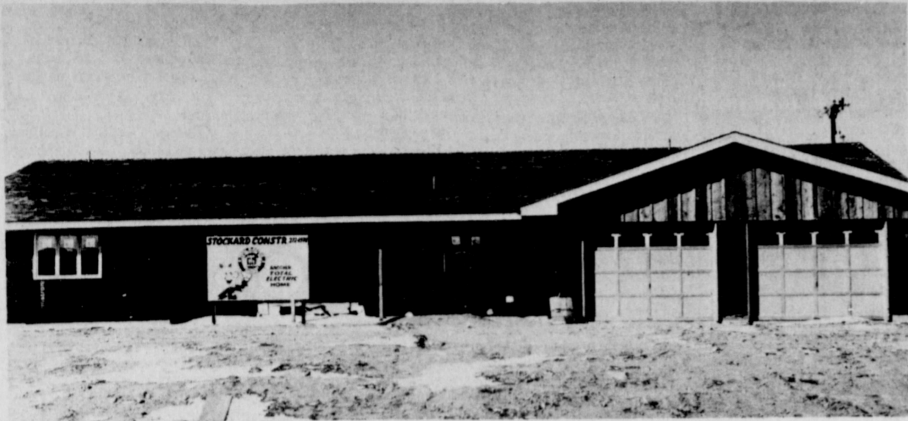
ANOTHER NEW HOME ON 20th...This new home is being constructed on 20th Street and Avenue G in the Richland Hills Addition. Several new homes have been constructed in this same area this year.
