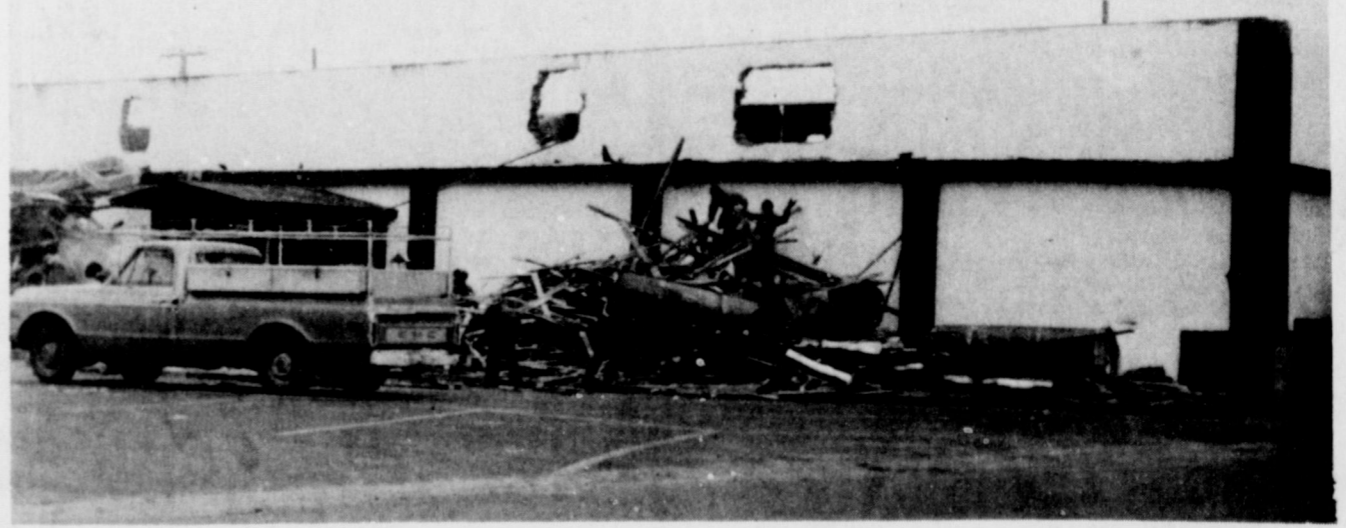
RECONSTRUCTION UNDERWAY...Remodeling of the XIT Steak House which recently suffered extensive damages due to fire, has been underway for sometime. At this time, the top roof
