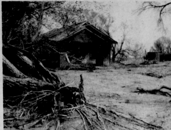
TORNADO EVIDENCE --This large tree, in the foreground, was uprooted by the force of a twister which swooped down on the Larry Davis home northeast of Muleshoe Sunday night. The porch columns were twisted out, windows blown out and the house looked as if someone had taken large buckets of mud and tossed them all over the outside of the home.
