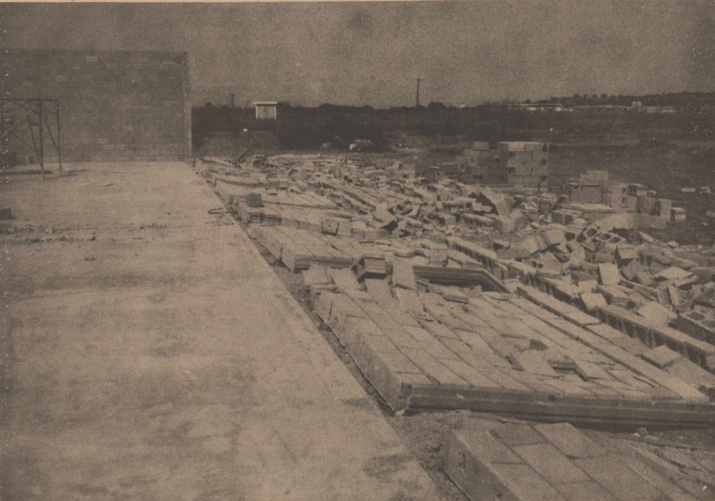
100 FEET OF CONCRETE BRICK WALL FELL VICTIM TO HIGH WINDS HERE MONDAY -- The wall was blown off the concrete foundation from one end of the building to the other Monday morning when winds were gusting to 50 miles per hour. The construction site is located behind the Arco Station on Ave. D.
