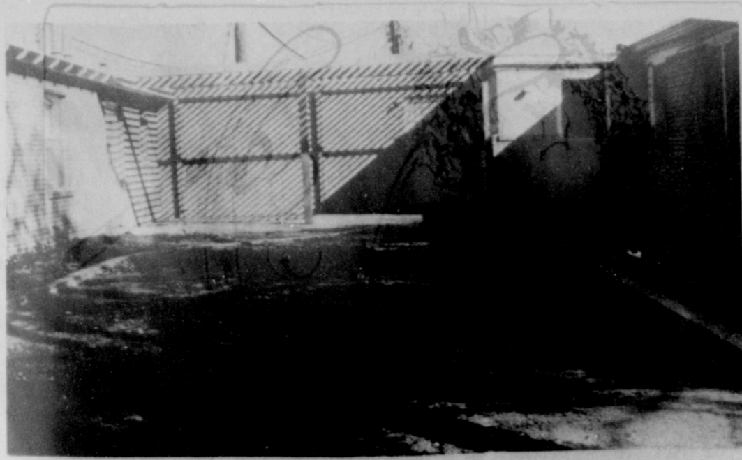
PATIO NEARS COMPLETION --In order to provide a spacious patio for patients and residents of the Muleshoe Nursing Home, work has been underway at the nursing home for the past several months. The patio is nearing completion at this time.
