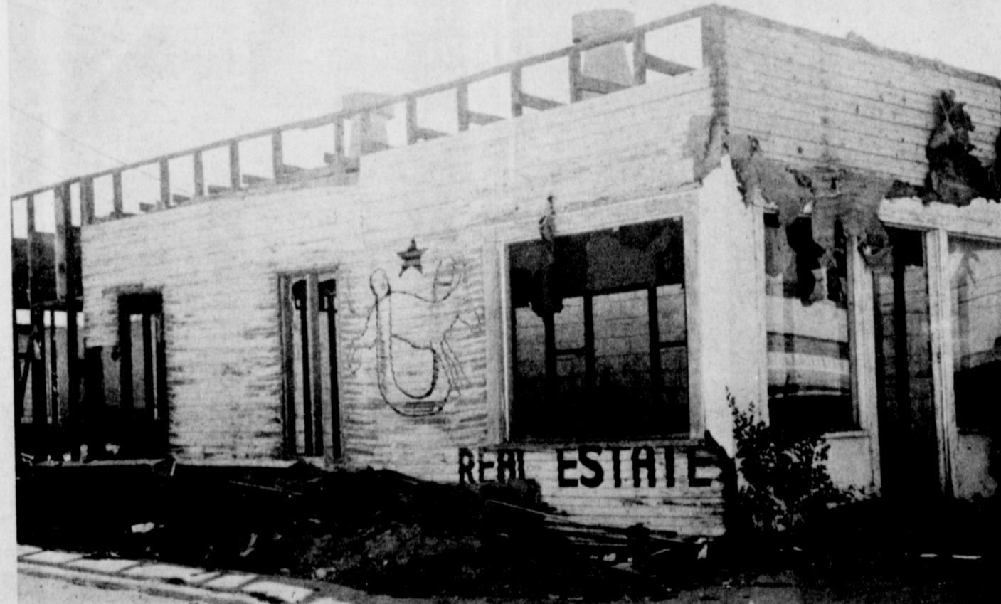
GOING--GOING--NEARLY GONE--Workmen are busy demolishing this old Muleshoe landmark. The building was constructed among the first permanent buildings in Muleshoe by the late R.L. Brown, who had the first mercantile store in Muleshoe. It is presently owned by his brother, D.P. Brown of Lavon. For several years, the building housed a real estate
