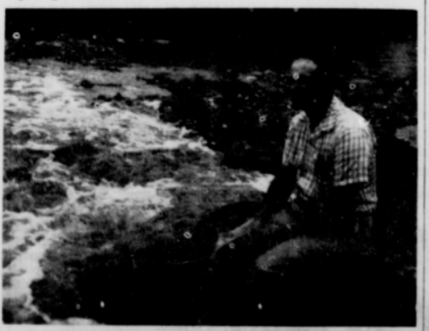
SITE 10 — Floodwater being released orderly into Pecan Bayou through 24-inch spun concrete reinforced pipe. Clayton Anglin, Soil Conservation Service Construction Inspector, of Baird, examining "draw down" pipe, just after 5-inch rainstorm on drainage area.
