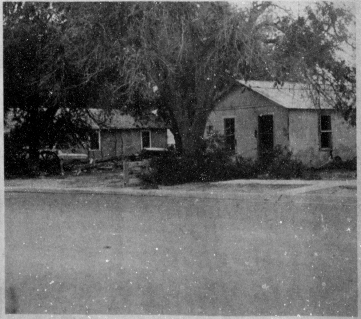
ABANDONED AND FALLING---- These two houses pictured are abandoned near Highway 84. The windows are out, weeds and trees are overgrown and the doors yawn wide on their hinges. These are just two of the spots noted that should be cleaned to help beautify our town.
