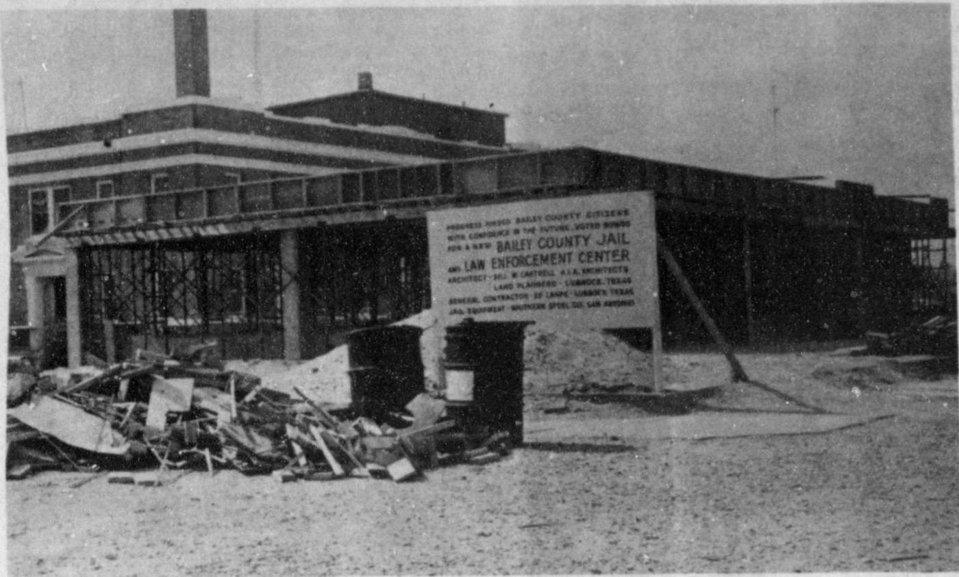
NEW CONSTRUCTION WELL UNDERWAY--With good weather for the most part during the past winter, the construction on the new City-County Law Enforcement Center is well underway. When the center is completed late this summer it will contain the new jail, and facilities for the city, county, state and justices of the peace. Construction shown in the picture above is the new jail which will be on the East side of the building.
