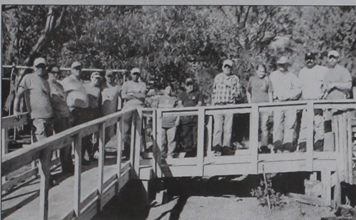
The Texas Ramp Project and volunteers led by the Clarendon United Methodist Youth build this handicapped ramp in Lelia Lake Saturday. The group also constructed a ramp at a home on Goodnight Street in Clarendon.
