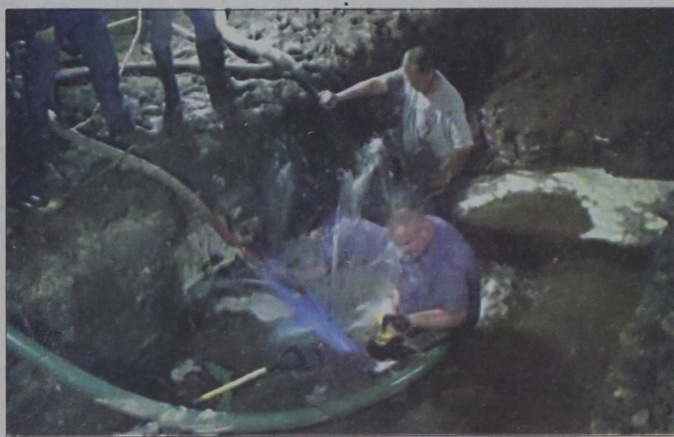
City workers Jeff McKee (white shirt), Coby Broughton (obscured by water), and Brandon Moody work to repair a ruptured line Tuesday evening, December 4.
