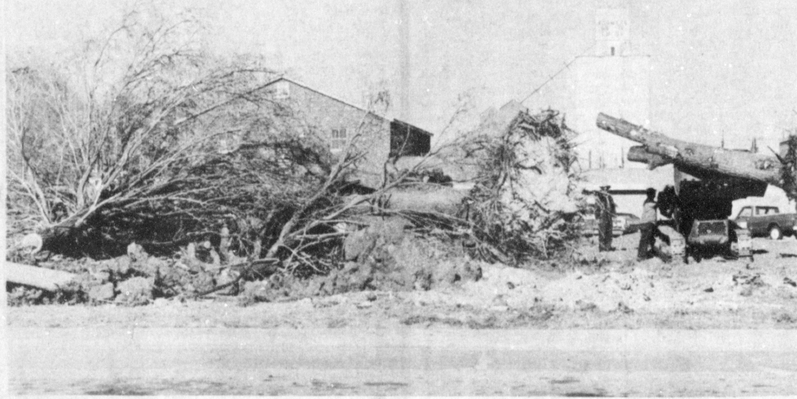
LAND MARK GIVES WAY TO PROGRESS--As the bulldozers began to clear the northwest corner of the courthouse square, making way for the new law enforcement center. The $175,000 center will have floor space of 4,000 square feet on the ground floor and another approximately 2,000 square feet in the basement.
