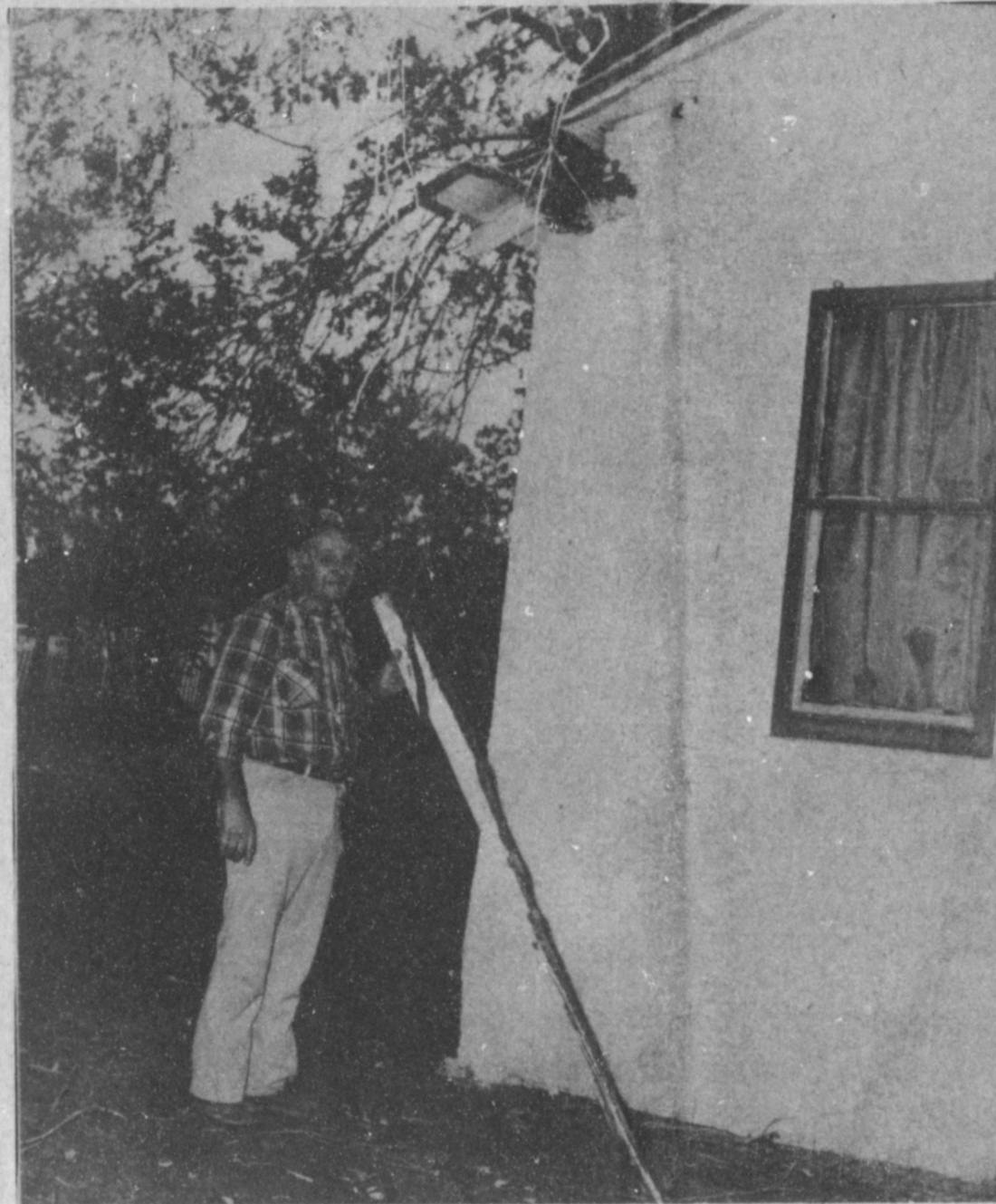
LOOKING OVER THE DAMAGE--Lester Elmore holds a two by four that was knocked from the edge of his house by an electrical storm in Muleshoe Wednesday afternoon. Above his head is a large hole in the roof and corner of the house from a bolt of lightning. A scorched and blackened area shows where a fire started, but was apparently extinguished by the heavy rain that accompanied the storm. The Elmores were not home when the lightning struck. Clocks were stopped in the home at 2:30 when the electricity went off.
