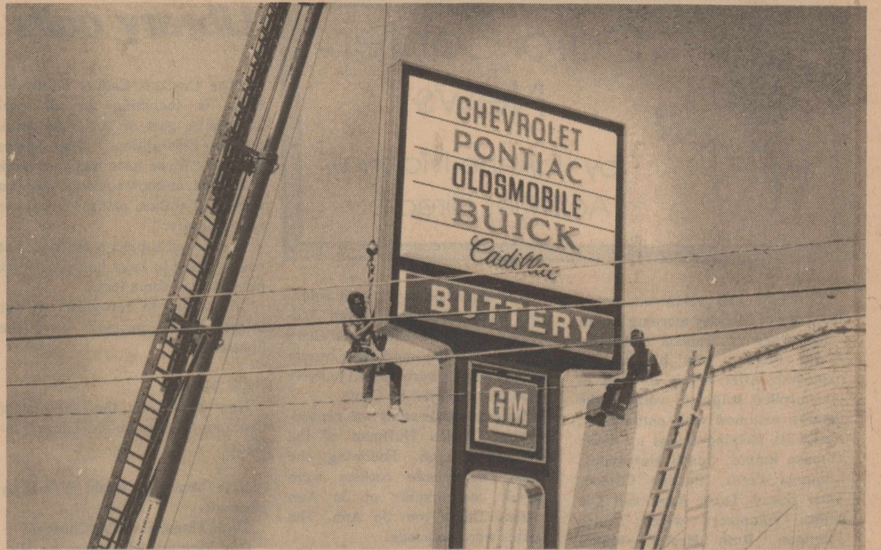
The name portion of the sign at BATTERY Motor Company was changed from L-B Motor Co. by daring
