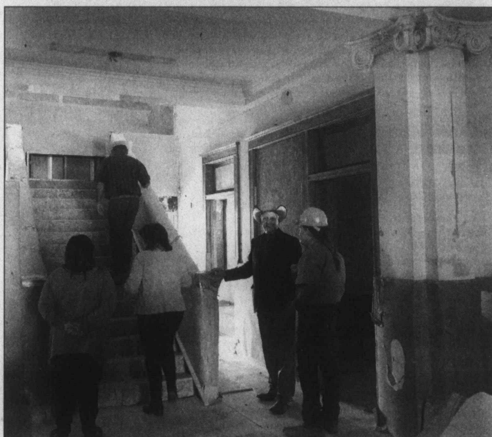
Let's look up here ... Commissioner John Hawthorne heads up the first floor stairwell of the county courthouse as Lynn County Judge Mike Braddock (at right) visits with the construction superintendent, Jerry Kissling, and other county officials look over the work in progress in the restoration project. (LCN PHOTO by Juanell Jones)
