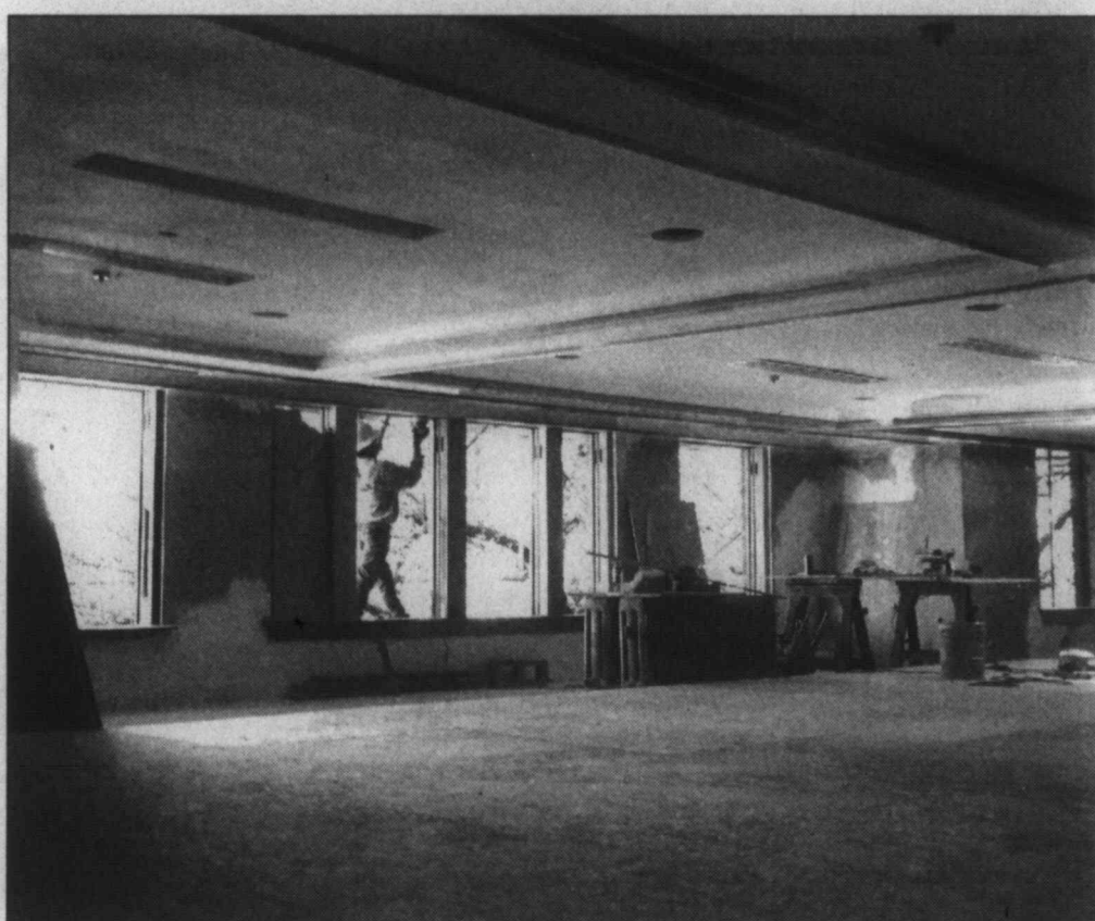
Work progressing ... A worker continues restoring the window framing in the Lynn County Courthouse on the third floor level, inside the district courtroom balcony area. The flooring here is actually a temporary plywood floor over the balcony seating area, to allow workers access to the ceiling. (LCN PHOTO by Juanell Jones)
