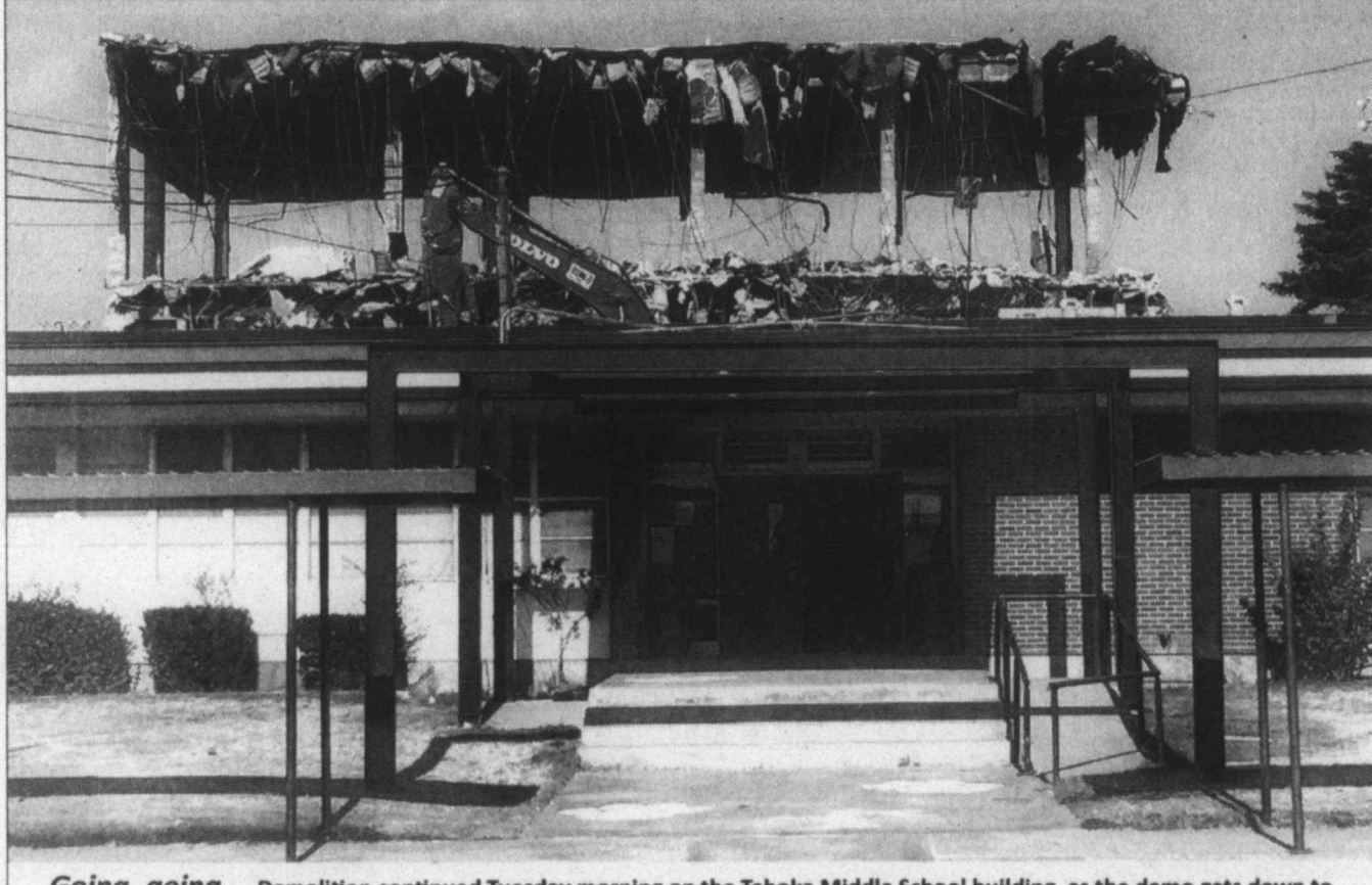
Going, going ... Demolition continued Tuesday morning on the Tahoka Middle School building, as the demo gets down to the basic framework holding up the building. It won't be long before the building is gone. (LCN PHOTO BY Juanell Jones)
