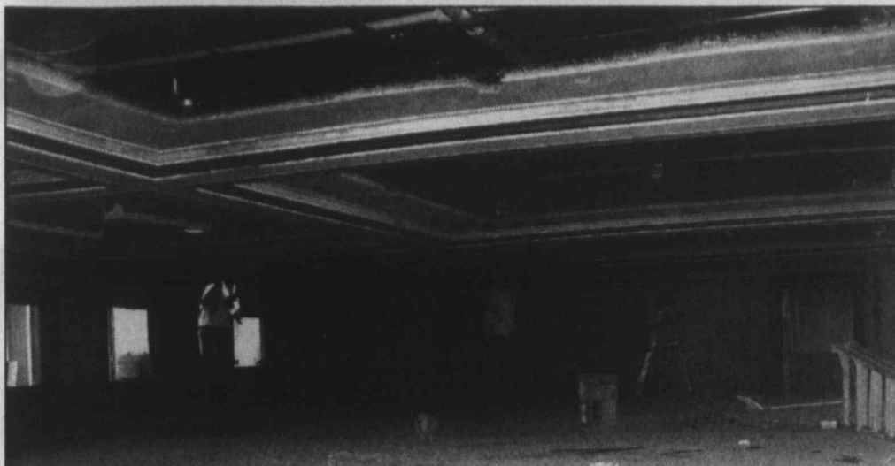
District Courtroom ... Lynn County's District Courtroom is having the original ceiling recreated during the courthouse renovation, which had long been covered with a dropped ceiling when the courtroom balcony was sealed off many years ago. Workers are standing on a makeshift ceiling placed in order to access the high ceilings here. When finished, the balcony area will once again be open for audiences. Note the original goldleaf scrollwork near the ceiling around the walls, which is also going to be restored. (LCN PHOTO by Juanell Jones)
