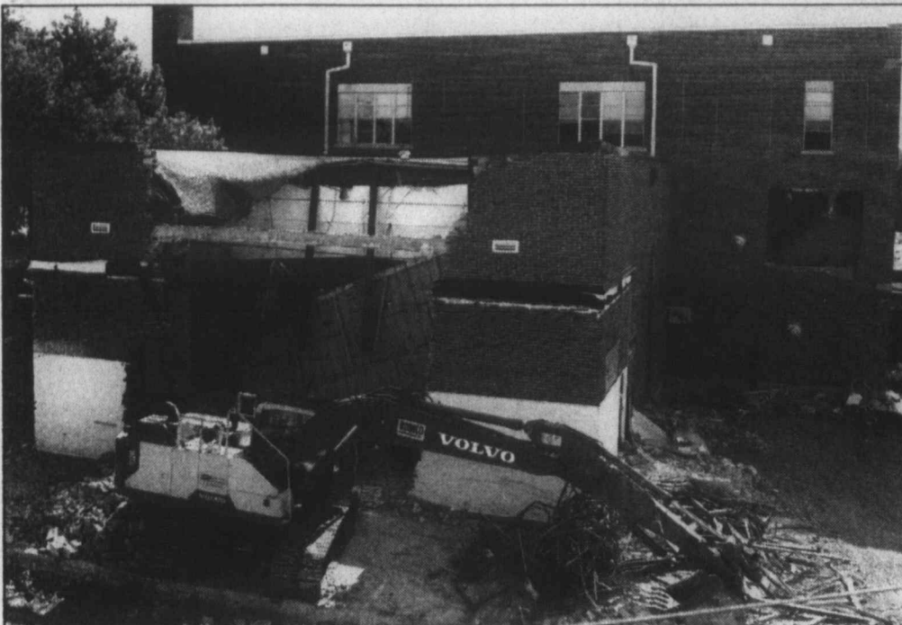
And the walls came tumbling down ... Demolition of the three-story Tahoka ISD building continues, with this picture showing the walls tumbling down on the back side of the auditorium, as well as the removal of the exterior fire escape from the middle school building. More has been done since this photo was taken last week. (LCN PHOTO by Pam Elrod)
