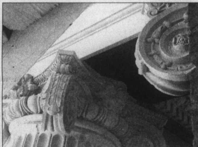
An exact replica ... The intricately scrolled masonry caps that sit atop the stately columns surrounding the Lynn County Courthouse have all been recreated with exact replicas during the renovation process. The original 102-year-old masonry had deteriorated to the point where it could not be repaired. (LCN PHOTO by Juanell Jones)
