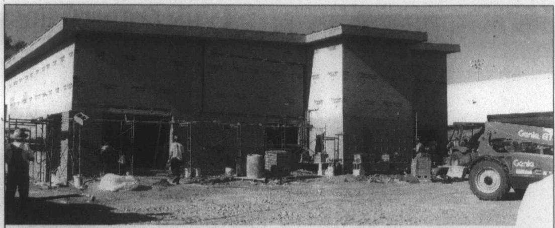
New auditorium ... Construction work continues on the Tahoka ISD campus, where a new middle school building and separate auditorium are being built. Pictured here is the auditorium, situated on the high school grounds in front of the THS gym. Workers have begun bricking the new building. The new auditorium is expected to be completed for the 2018-19 school year. (LCN PHOTO by Juanell Jones)
