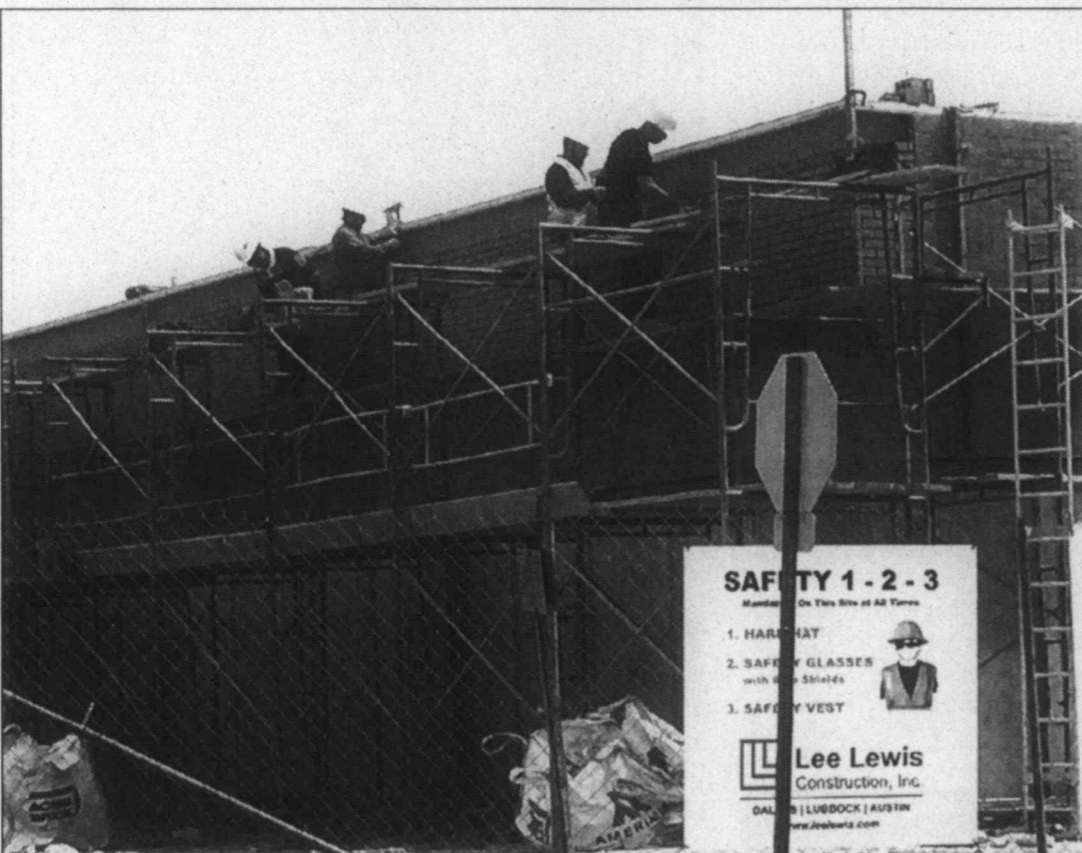
Work coming along ... It's beginning to look more like a school building, as the brick work nears completion on the new middle school classroom facility on the Tahoka ISD campus. Across the street, the framework is up for the new auditorium, which is situated in front of the THS gym.
