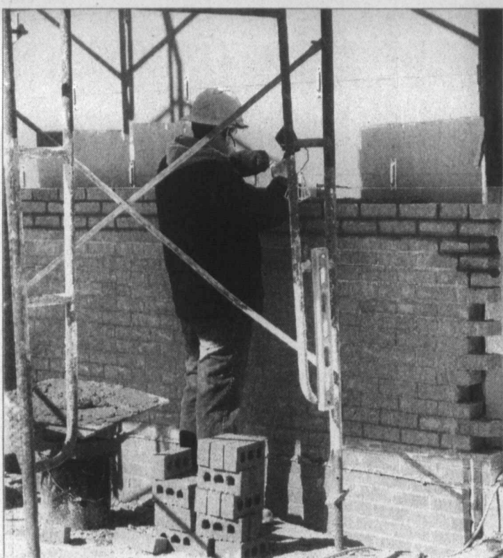
Brick work ... Construction work continues at Tahoka ISD, where the brick work is underway on the new middle school building, located across the street from the THS gymnasium.
