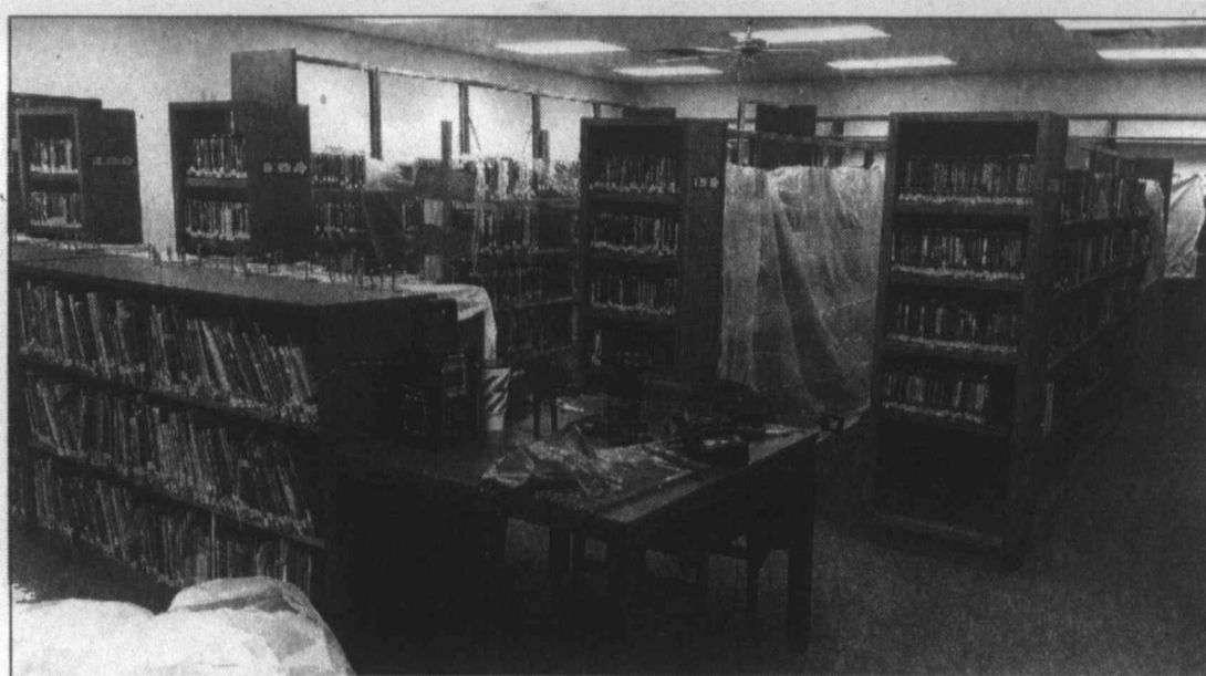
A change is coming ... Construction for expansion inside the City-County Library in Tahoka has begun. More construction will happen beginning October 30.
