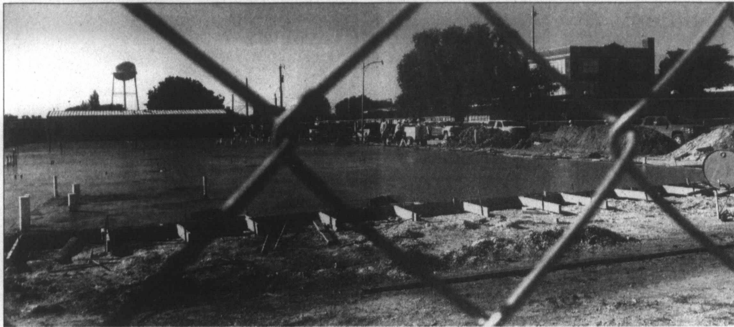
Progress in school construction ... The concrete foundation for Tahoka ISD's new Middle School was poured last week, as progress continues in the TISD construction project. The new middle school is located across the street from the THS gymnasium, on the corner of N. 4th and Ave. P. (LCN PHOTO by Juanell Jones)
