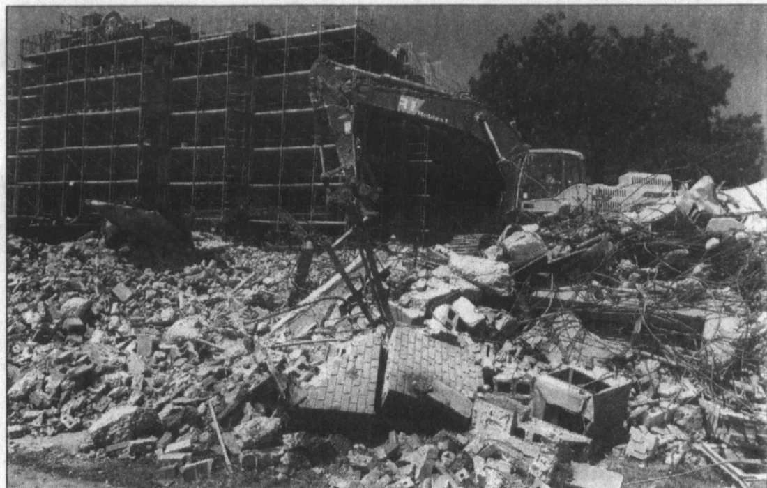
Jail house rock ... Nothing but concrete rocks and other debris remain from the old Lynn County Jail that was located on the southeast corner of the county courthouse, as the old building has been demolished as part of the courthouse renovation project. The debris is being cleared this week. The former jail was built in the early 1960s, but since about 2002 had only been used for storage, since the new jail was built out on Hwy. 380. New wells for the courthouse's new geothermal heating/cooling system will be dug here, and then the area will be covered in grass. (LCN PHOTO by Gary Jones)
