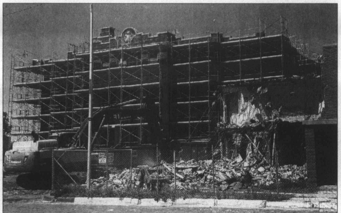
Coming down... Construction crews are in the process of removing the old Lynn County Jail at the courthouse as part of the restoration project. (LCN Photo by Pam Elrod)
