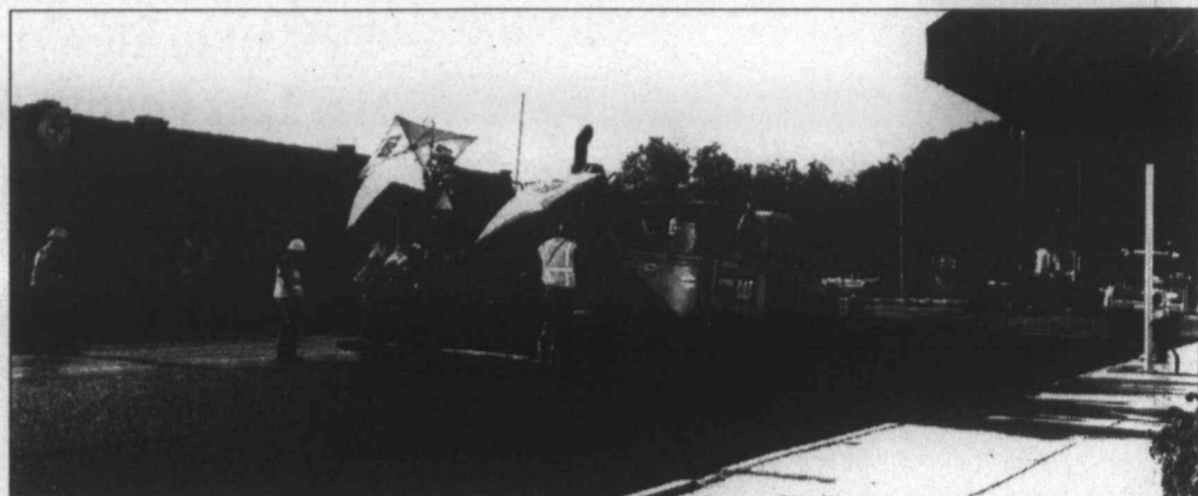
Main Street gets new paving ... Main Street, from the courthouse to the northern edge of Tahoka, was getting new pavement last week, as part of TxDOT's agreement with Lynn County and the City of Tahoka. This is the route for Loop 472 in Tahoka, that comes from the US 87 exit through Tahoka and curves past the courthouse to go on to access US 87 on the south edge of town. Loop 472 will not exist much longer, however, as a portion of the street that curves through courthouse grounds will be removed as part of the Lynn County Courthouse renovation project. The square will be restored to include the memorial triangle, and traffic will be routed around the courthouse when complete. This week, TxDOT had moved on to repave the rest of Main Street. (LCN PHOTO)
