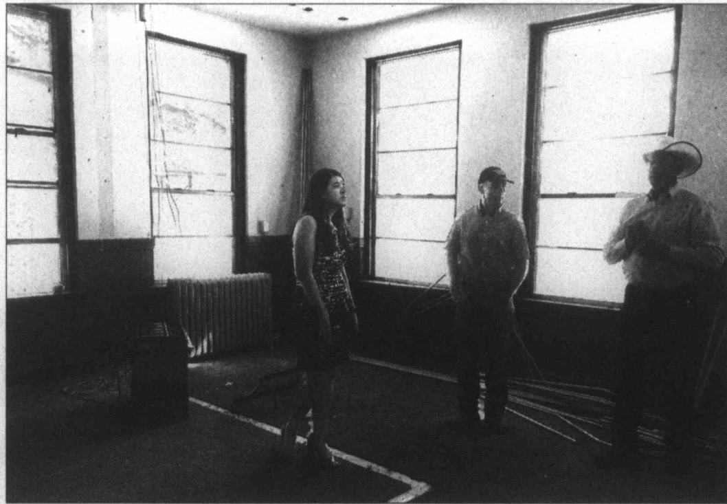
Renovation underway ... On Monday, after the Lynn County Commissioners meeting, the County Judge, Commissioners and several other county officials ventured into the Lynn County Courthouse to see how the renovation project is getting underway. Construction workers have covered the original tile floors and marble stairways to protect them during the project, and repair of window facings, electrical and other work is just beginning. The 101-year-old courthouse, until now, was heated with the original floor and wall radiators using the original boiler in the basement. With the renovation, a new geo-thermal heating and cooling system will be installed, and most of the old radiators will be removed. Some will be placed in the public areas of the courthouse for historical value, but will be for looks only. It is anticipated that an auction may be held at a later date to allow the public an opportunity to purchase some of the other antique radiators, and possibly some other items that won't be used. (LCN PHOTOS by Juanell Jones)
