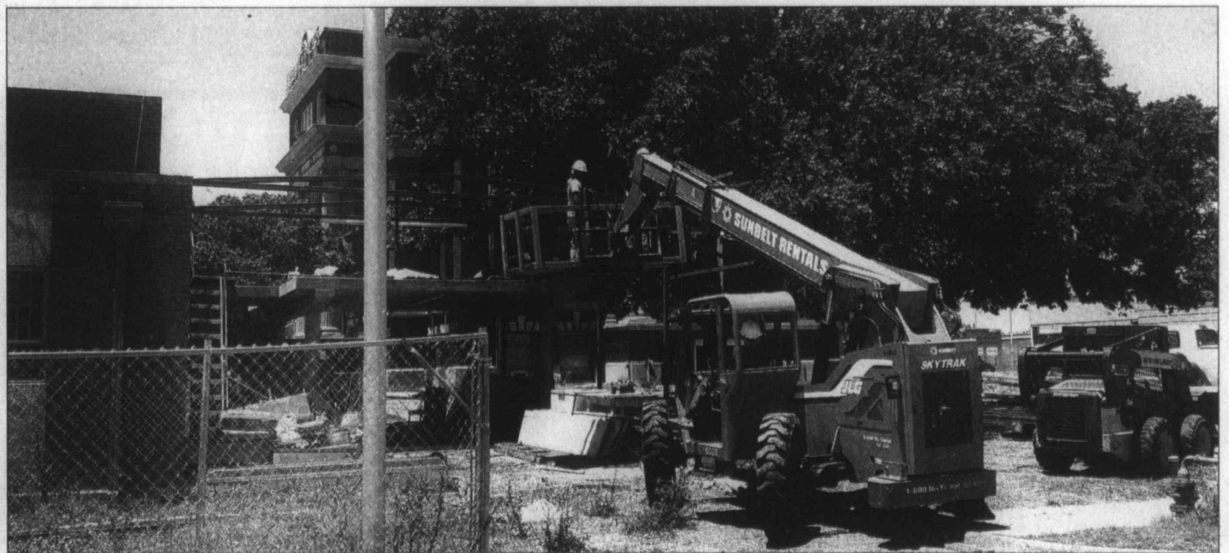
Sally port coming down ... Workers carefully dismantle the sally port at the old jail just east of the Lynn County Courthouse as part of the current renovation project for the courthouse. County Judge Mike Braddock told the News that the old sally port will be reassembled and used at the Lynn County Precinct 2 barn here in town. (LCN photo)
