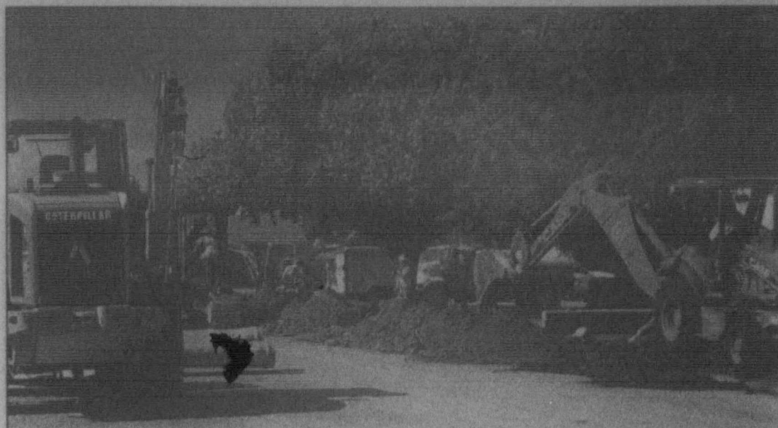
Waterline project ... Progress continues on the City of Tahoka's waterline replacement project, which began in mid-October. In this photo taken last Thursday, workers were digging trenches and laying pipe along the front yards on North 6th Street, between Ave. L and K. City residents are reminded to use caution in work zones, and to speak with construction workers if there is an issue accessing their property. (LCN PHOTO)
