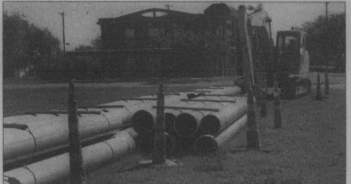
Pipeline ready ... Tahoka citizens will see blue pipes stacked around town, such as this on Ave. P and N. 6th, where the city's waterline replacement project is expected to begin this week. (LCN PHOTO by Pam Elrod)
