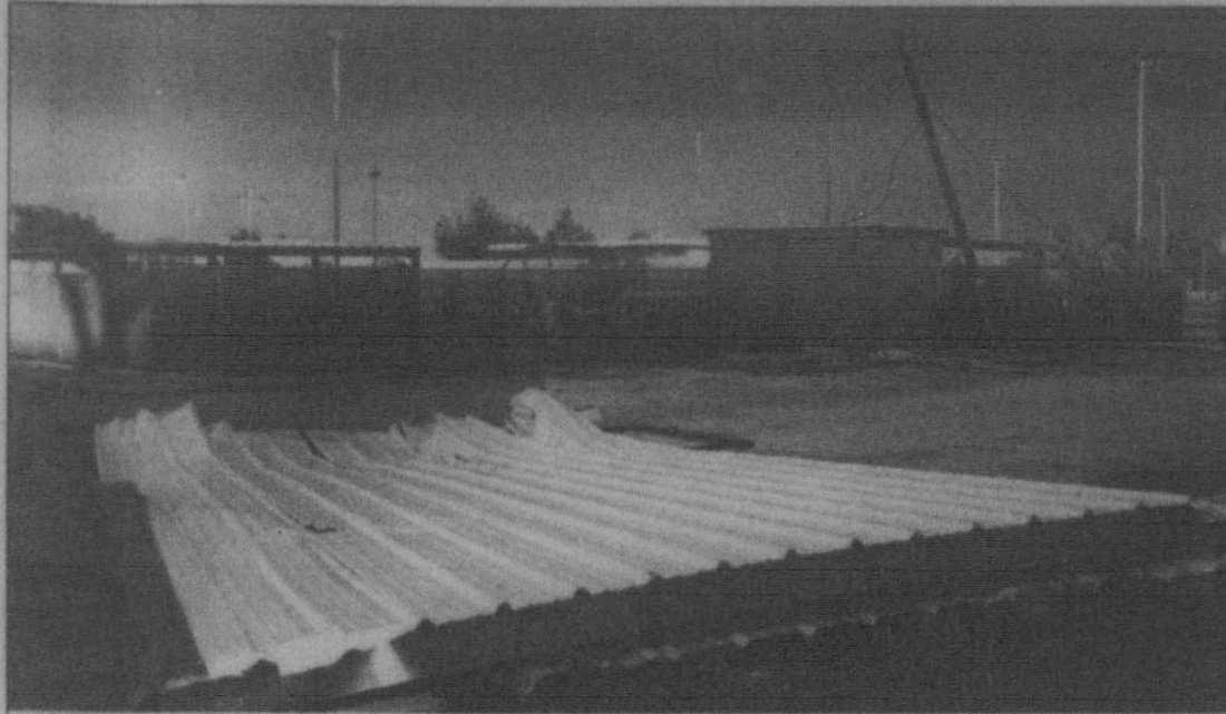
Not where that belongs ... The metal roof, with framework and all, was lifted off the concession area of the Tahoka City Pool last Thursday evening during some strong wind gusts during a passing thunderstorm. No damage was done to the concession or pool area, but Xcel Energy did have to come and repair a pole and line that was pulled over. The pool is open for business as usual. (LCN PHOTO)
