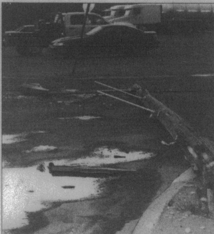
Pole down ... This pole snapped at the corner of Main Street and N. 3rd during some strong wind gusts in Tahoka during a passing thunderstorm Thursday evening. Xcel Energy repaired the pole. (LCN PHOTO by Juanell Jones)
