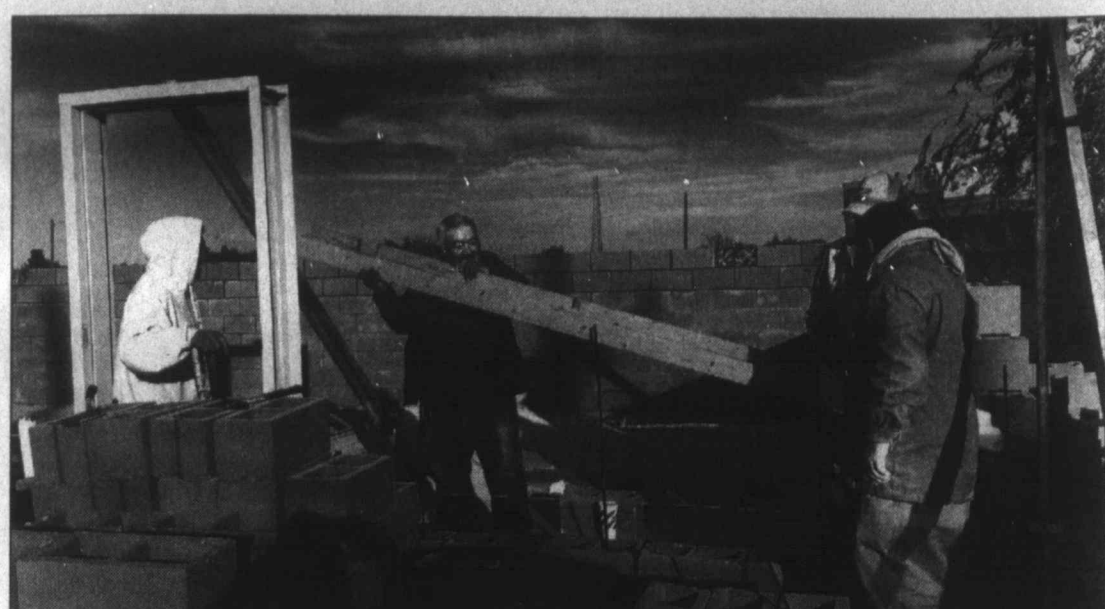
Walls going up ... Concrete block walls were being erected last week on the addition to the Lynn County Animal Shelter, located on the southeast corner of the square in Tahoka. The new addition will connect to the current facility, and will include laundry/restroom facilities, as well as space for medical supplies, a small office, cat facilities, storage, and medical treatment area. The work is being done by Eddie & Ruddy Masonry. (LCN PHOTO by Juanel Jones)
