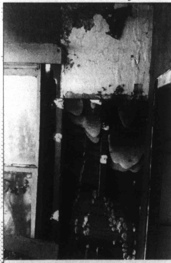
Not what you want in the walls ... This extremely large bee hive covered the entire wall from floor to ceiling before Tim Pledger removed some of the hive inside an abandoned house in North 3rd. The bees were relocated to a new hive. (Photo by Tim Pledger)
