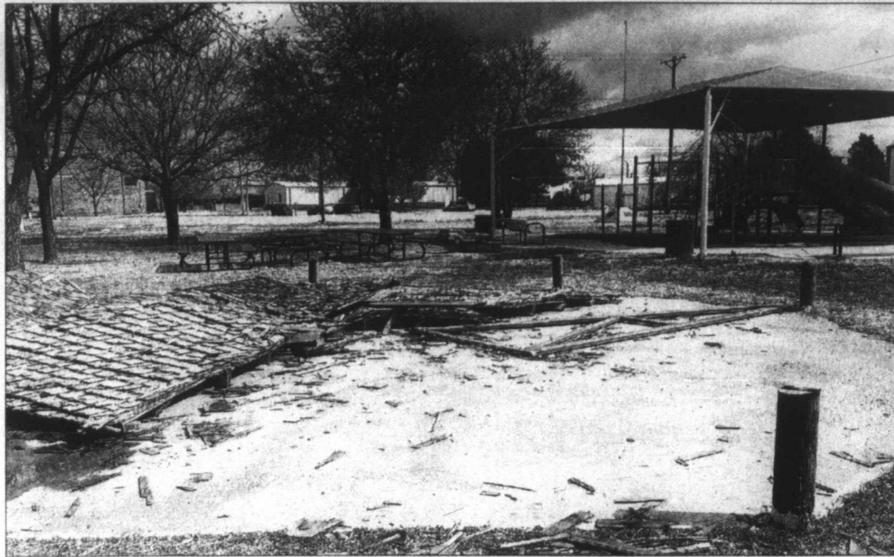
Old for new ... The old wooden roof over the octagonal gazebo in the city park was removed this week, in preparation for new metal roofing. It's a renovation project undertaken by the A.C.T. Board (Advancing the Community of Tahoka) using funds collected through a half-cent sales tax.
