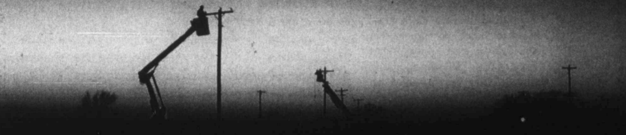
This is part of Lyntegar's Lamesa crew working west of King Mesa Gin to repair lines. The lights on the right are from a tractor. "Many of the generous farmers in our service area assist our crews by pulling us with tractors when the conditions call for it. Thanks to all the farmers assisting our crews!" said a Lyntegar spokesman.
