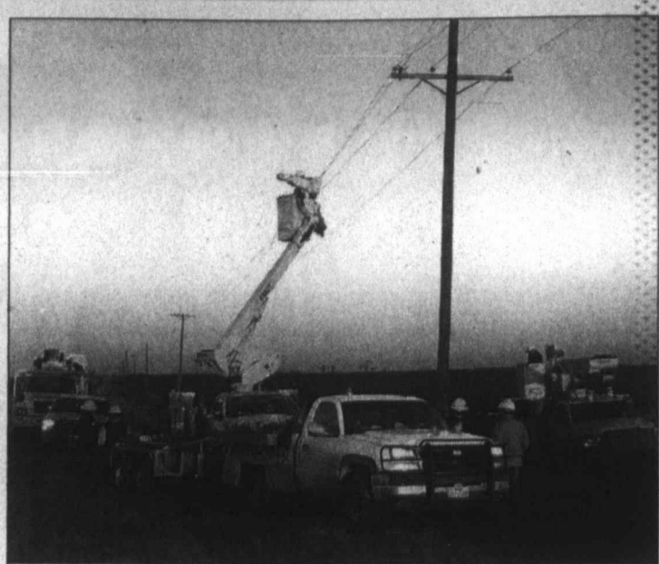
Team effort ... Lyntegar Electric Cooperative's Seagraves crew is pictured here as they repair electrical lines near Flower Grove on the Martin/Dawson county line. Approximately 500 poles were down, and 2,500 cross arms damaged or down in Lyntegar's rural service area after the New Year's icy weather, causing power outages in Lynn, Borden, Dawson and Gaines counties.
