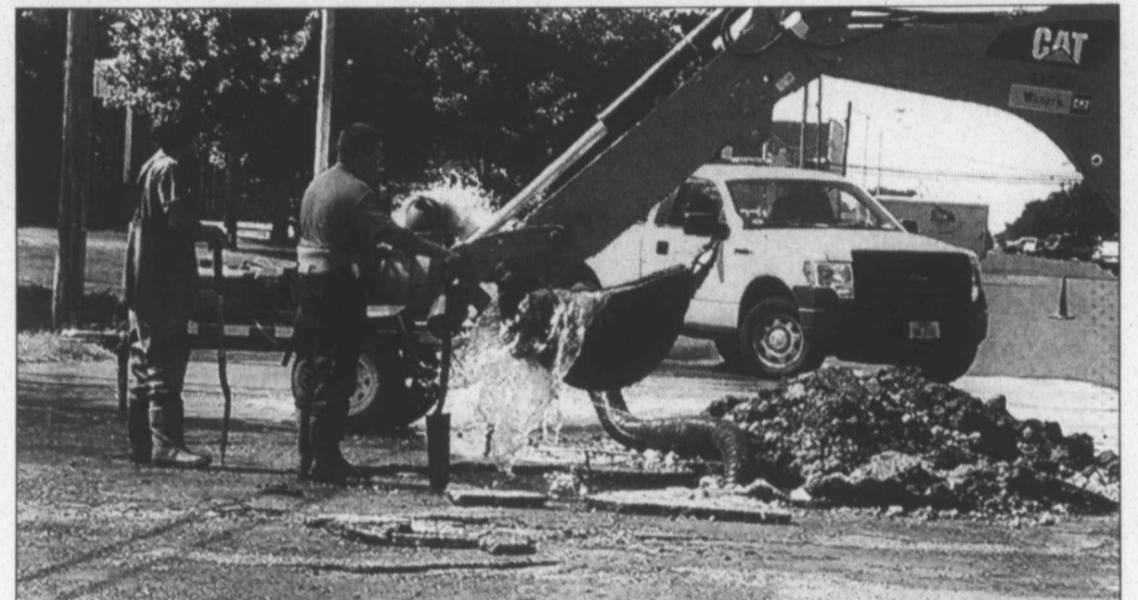
Water break ... City residents were without water for a brief period last Wednesday morning, as city employees worked on a large break in the waterline beneath the intersection of N. 1st and Ave. J in Tahoka, just behind the Lyntegar Electric Cooperative office. A boil water notice was initiated until the water could be tested. City workers pictured here are Candalaria (Candy) Frausto and Michael DeLeon.
