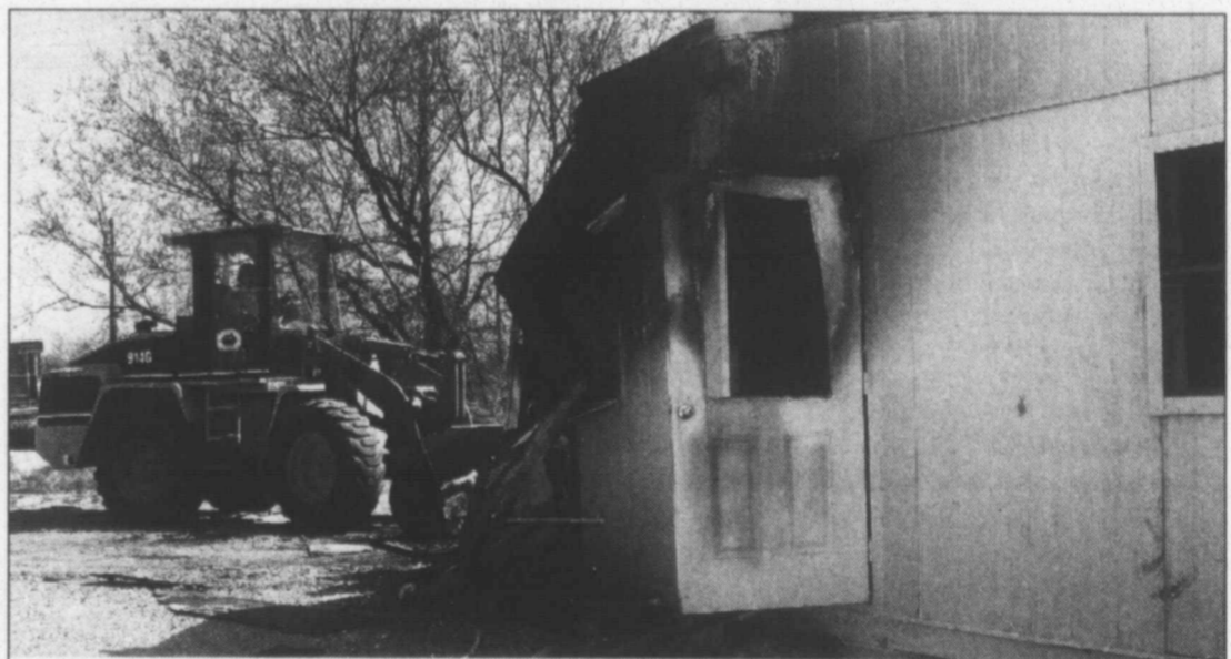
New beginnings... Workers are clearing off this building at the Lynn County Animal Shelter that was recently lost to a fire that claimed the lives of seven cats. To date, funds in the amount of $14,945 have been raised to help with construction of a new office/shelter. Also, Tahoka NHS and Student Council were able to raise $350 for the Lynn County Animal Shelter through the "Hugs for Pugs, Kisses for Kittens" fundraiser held recently.
