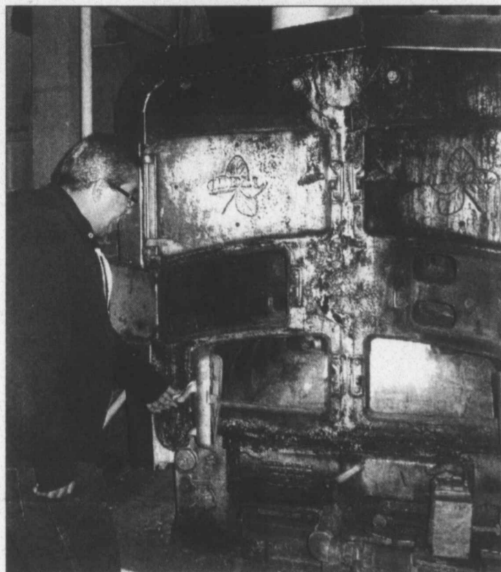
Still works ... Rigo Avila opens a door to look inside the original boiler at the Lynn County Courthouse, installed in 1916 when it was first built, which is still in service providing heat nearly 100 years later for the historical building that houses county offices. The behemoth iron box squats in the bowels of the building, with flames heating water to push steam through the pipes to the radiators that provide heat throughout the four-level building. Etched in the front of the boiler is a date: May 9, 1905. (LCN PHOTO by Juanell Jones)
