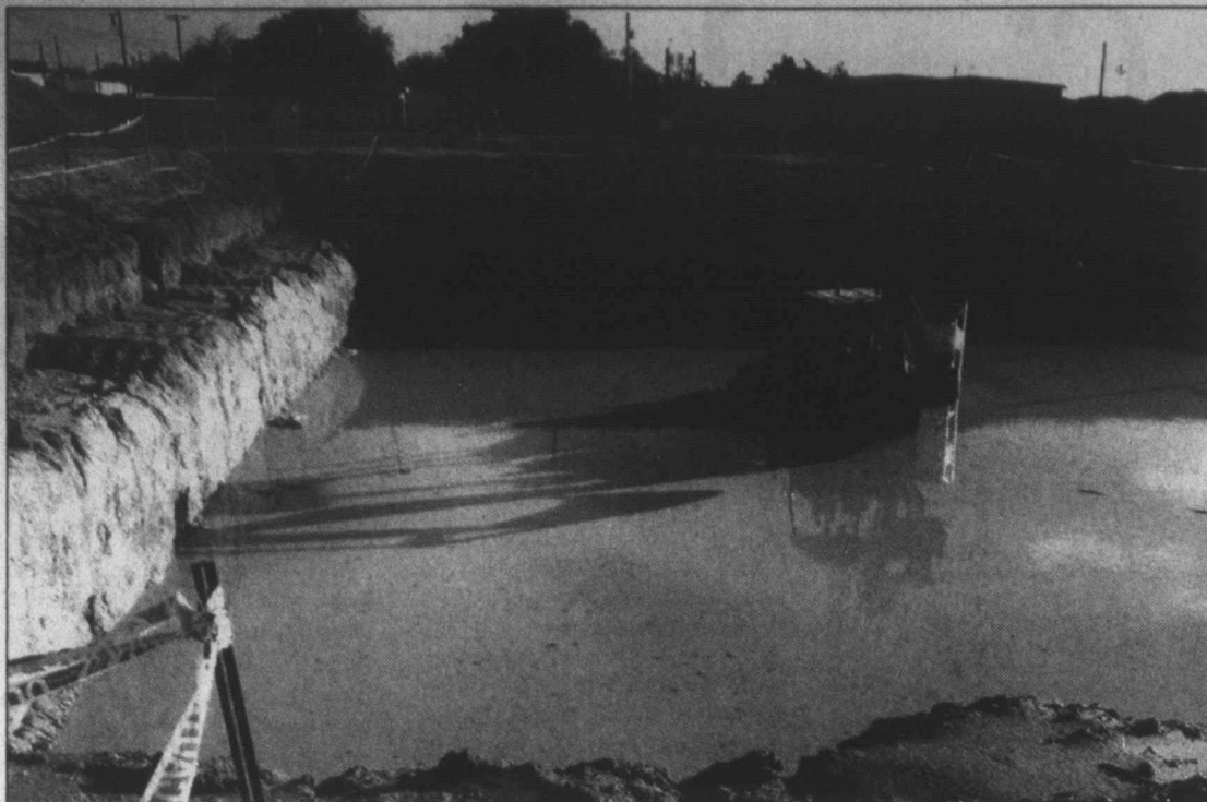
Mud pool... This photo, taken by Rusty Cook Tuesday morning following the thunderstorms that blew in Monday evening, is of the site of the future Lyntegar basement now under construction. The official rain total from Monday night was 2.45 inches.
