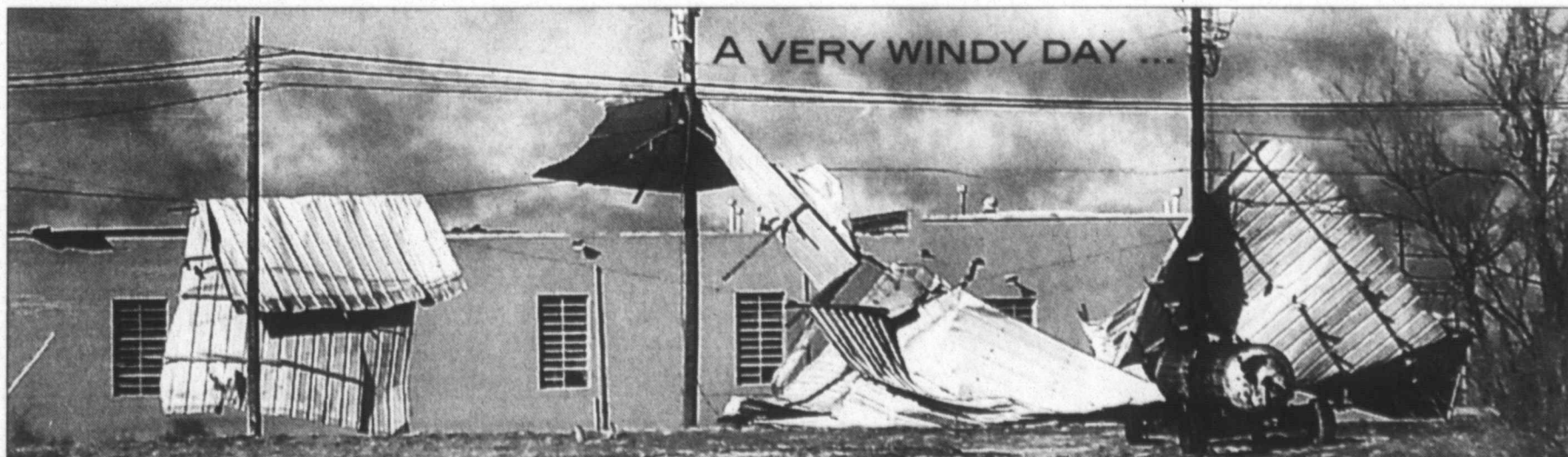
The wind won ... High winds Monday picked up the metal roof on the LCHD fitness center on Hwy. 380, peeling off large sheets of metal roofing and flinging them over power lines behind the building, looking almost like giant sheets hanging on a laundry line. Tahoka residents experienced a brief moment of power outage from the mid-afternoon incident. The winds were generated from a powerful blizzard that struck the northern panhandle of Texas Monday, but Lynn County mostly received blowing snow with no accumulations. Icy road conditions early Monday created some traffic hazards as well. (LCN PHOTO by Abraham Vega)
