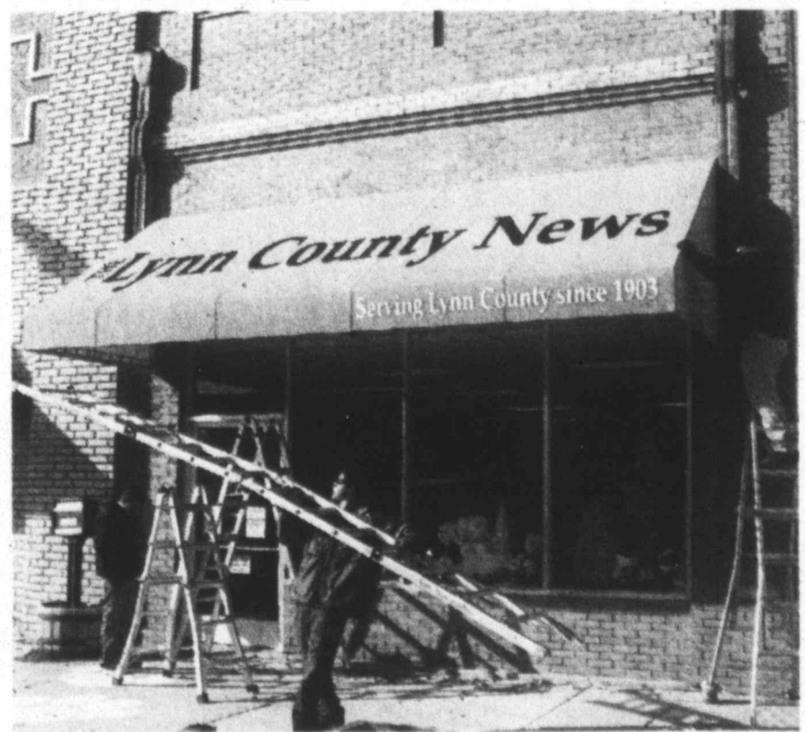
Our new look ... Workers put the finishing touches on a bright new awning and sign affixed to the front of The Lynn County News recently, replacing the decades-old metal awning that this summer's hailstorm redecorated with baseball-size dents. It's a new look for 2013 for the News Office, located at 1617 Main Street in Tahoka.
