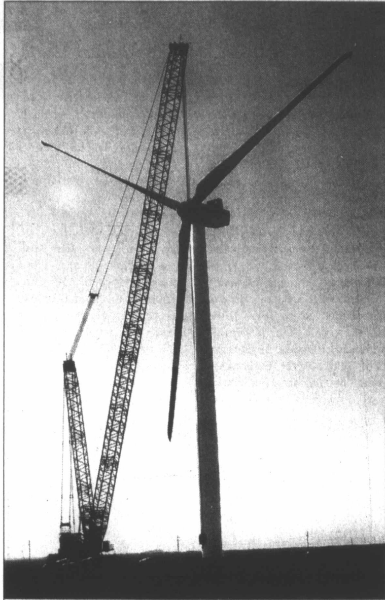
First one completed ... The first of 17 wind turbines was completed last week, at the Cirrus 1 wind energy project near Draw in southern Lynn County. The turbines are among the tallest in the United States, with blades measuring 185 feet towering high on a 270-ft. base. The 3.6 MW wind turbines will have the largest output per turbine of any in the US. The wind energy project is expected to be completed by the end of 2012. (LCN PHOTO by Gary Jones)
